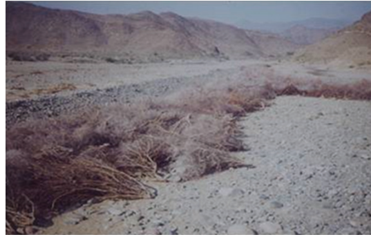
Image 3. Use of Brushwood to divert spate flows. Next to wood is a stone and soil structure. (Spate Irrigation Network International).
