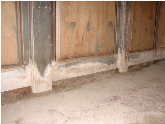
Image 16. Salt efflorescence on timber structure before conservation (Tinghsin Hote Foundation).
