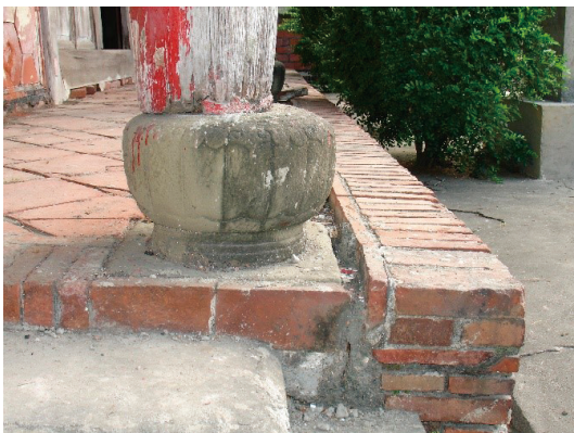
Image 17. Timber pillar misplaced on the stone pedestal and the cracking of the foundation due to distortion caused by moisture fluctuation (Tinghsin Hote Foundation).
