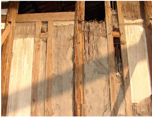
Image 26. The original bamboo wattle and daub wall that was in a state of degradation (Tinghsin Hote Foundation).
